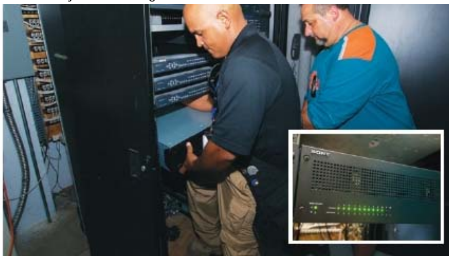
Aware Digital technician Adan Canuelas places a Sony SNT-RS3U chassis equipped with SNT-EX154 encoder blades (inset) into an equipment rack while Detective Juan "Johnnie" Villalobos interfaces with the system. The solution records at 30 frames per second.
